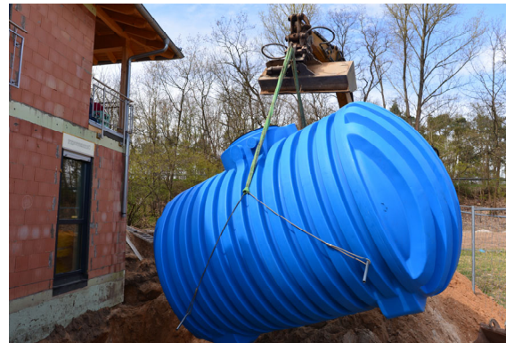
Regenwasserzisterne © Adobe Stock, Ilhan Balta
